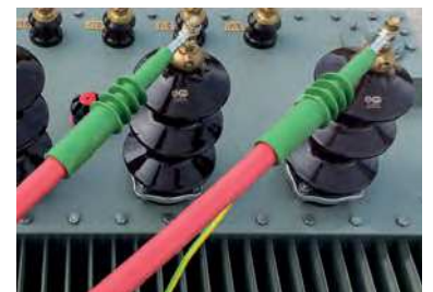
AIP20 as a transformer connection
